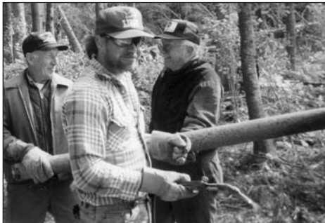
From left: Uno Issacson, Steve Stubenrauch and Mark Stubenrauch cut steel pipe uprights off old water tank at Mouth of the Gratiot clean-up.
